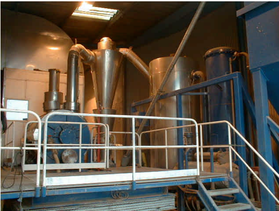
Figure 5 A diesel powered TCC installation.
