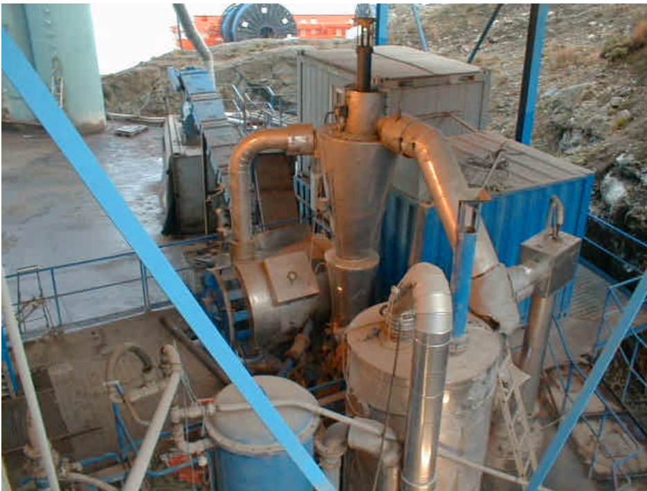
Figure 3 The TCC-450 kW installation operated by Soilcare AS.
